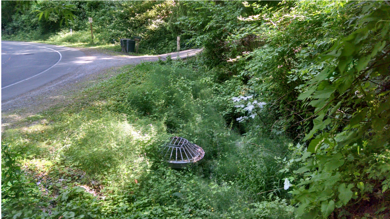
Photo: Type-2 catchbasin with beehive grate overflow conveys Stream A across and beneath East Mercer Way.
